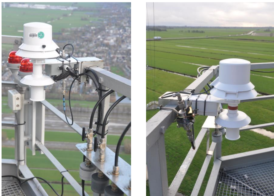
Fig. 4: Air inlets and filters at different heights in the Cabauw tower (27m and 207m).
